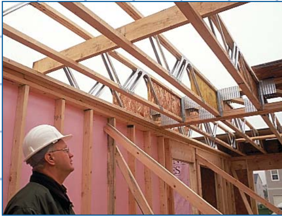
IF BRACING IS CUT OR ALTERED CONTACT YOUR SPACEJOIST TE REPRESENTATIVE.
